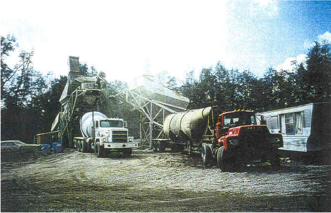
FIGURE 6 – TRANSIT MIX BATCH PLANT
